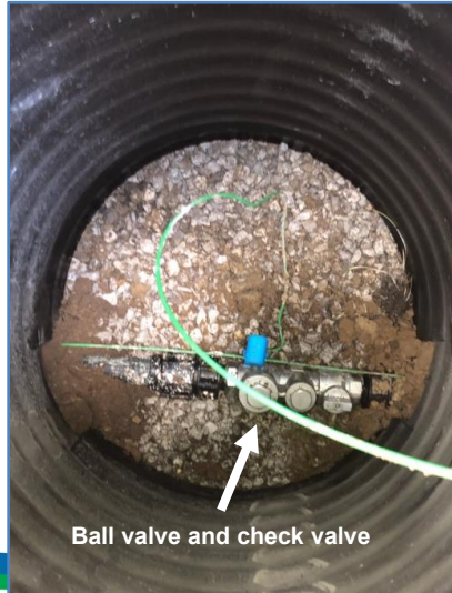
Pictured below: Inside of Service Box/Valve Pit
