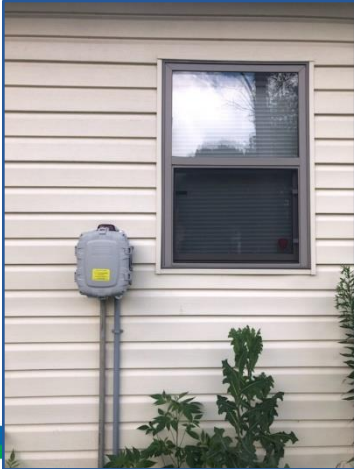
Pictured below: Installed Control Panel
