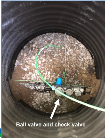
Pictured below: Inside of Service Box/Valve Pit
